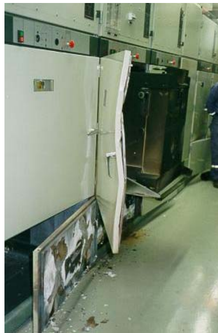
FIGURE 1: A cubicle damaged by arc short-circuit.
